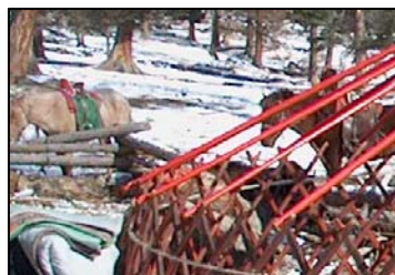
Loops attach the rafter poles to the lattice; the poles stick out slightly beyond the lattice.
